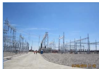
S.E. San José 500/220 kV
