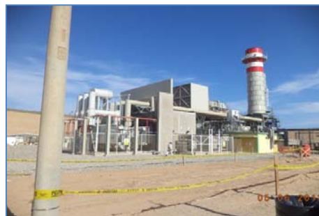
Turbina a gas (TG2)
