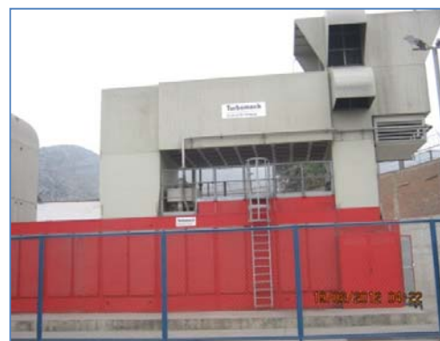
Turbina a Gas
