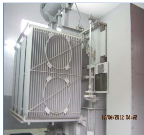
Transformador Principal 17/20 MVA 13,8/22,9 kV
