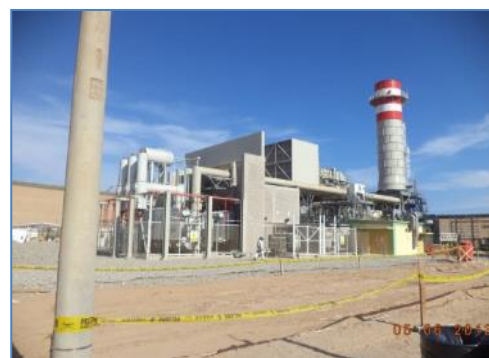
Turbina a gas (TG2)
