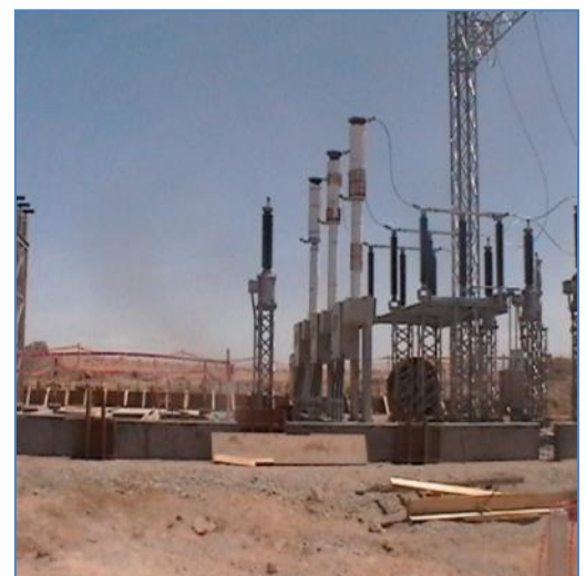
S.E. Central Panamericana Solar (23/138 kV)
