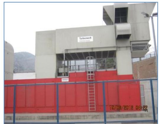
Turbina a Gas
