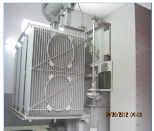
Transformador Principal 17/20 MVA 13,8/22,9 kV
