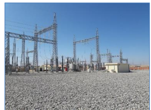
Patio 220 kV – TR 50 MVA – Patio 60 kV
