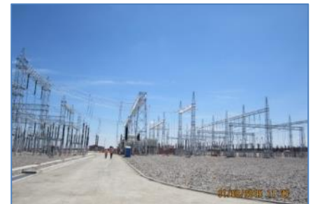
S.E. San José 500/220 kV
